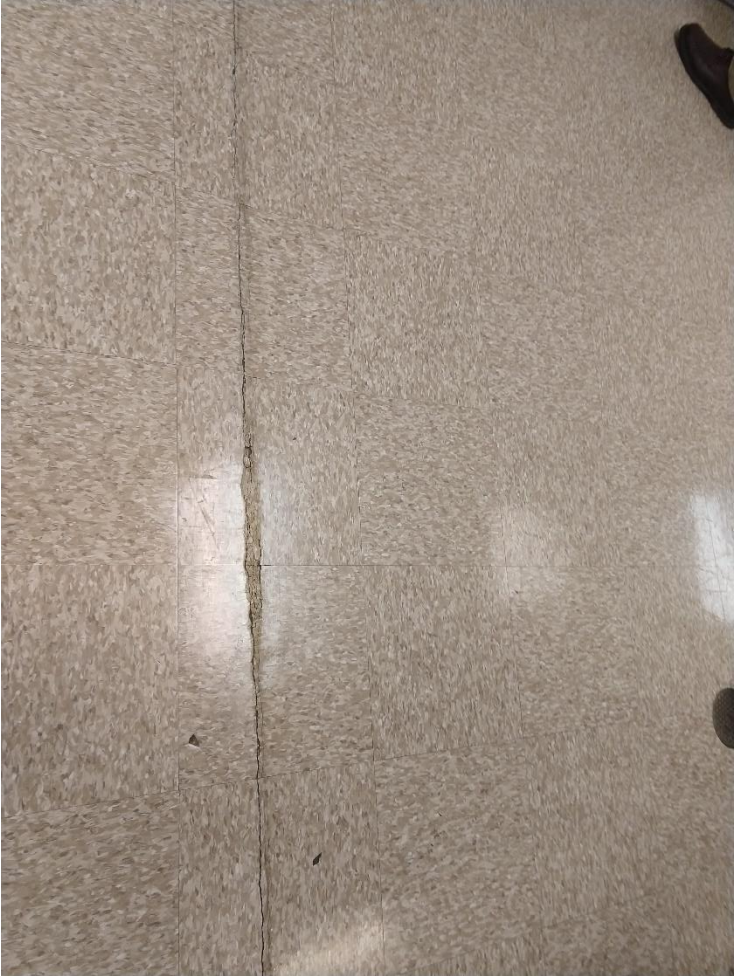
New Jail Addition - Unsettling
