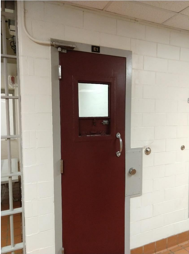
Door Not Compliant -Door Width
