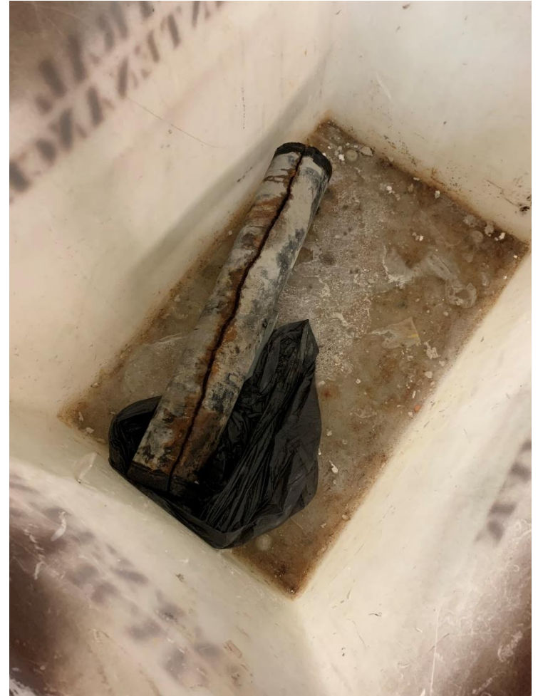
Plumbing – Pipe Breaking
