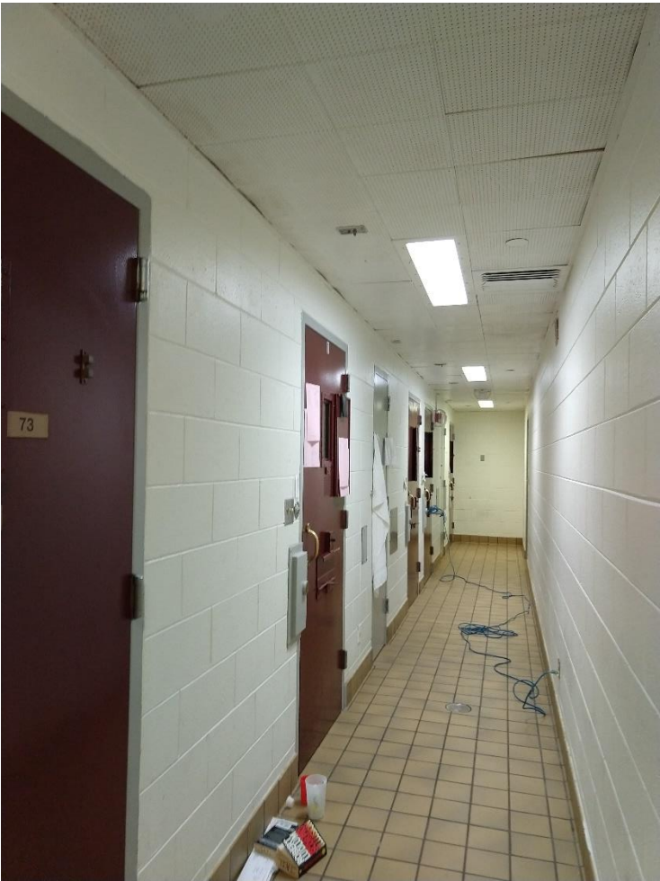
Time-Out Corridor -Electrical Cord Across Floor
