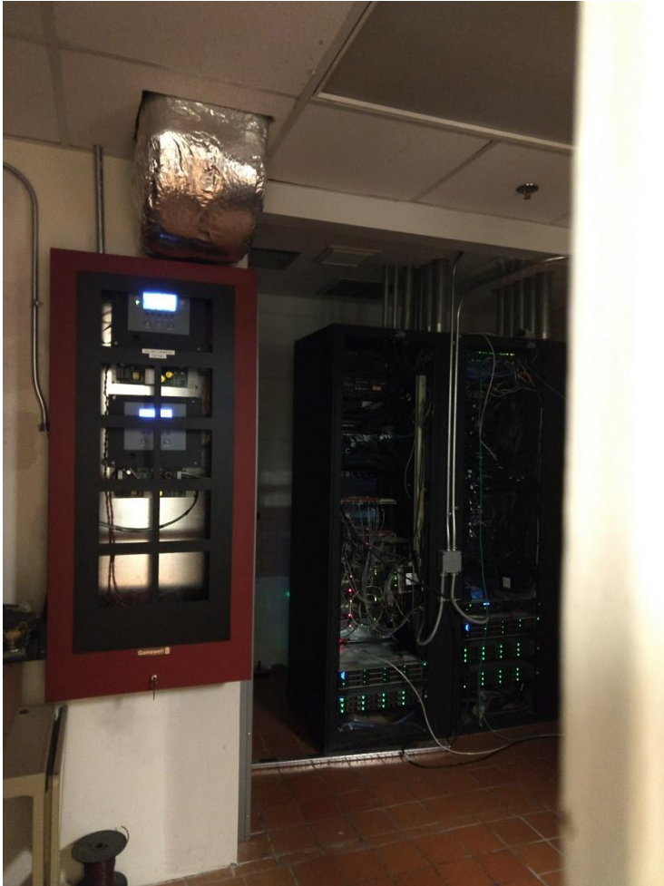
Jail – Security Electronics - Not in a conditional space
