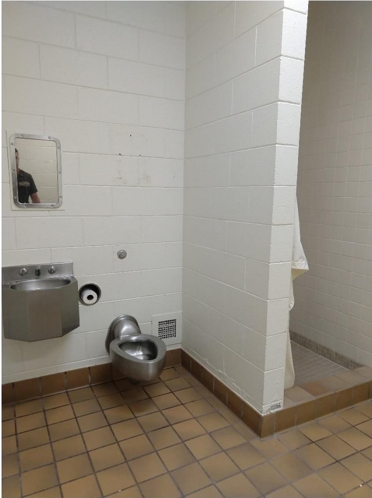
Detainee Toilet/Shower - Not Code Compliant
