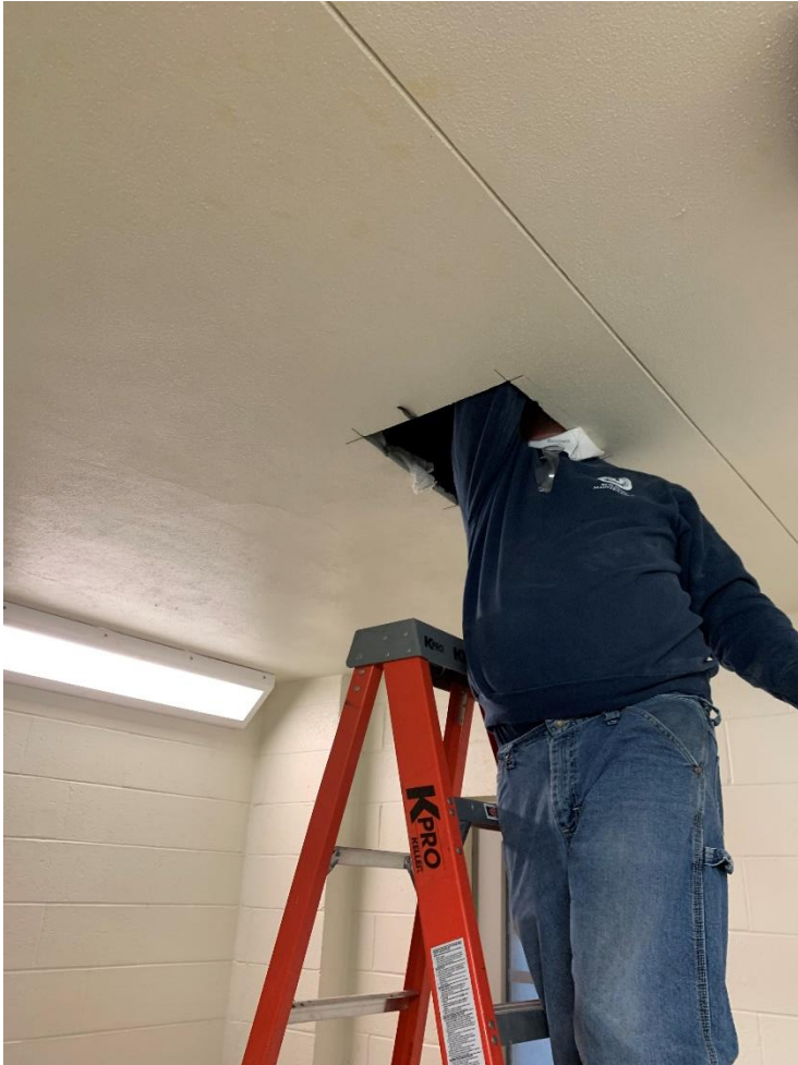
Plumbing – Pipe Breaking
