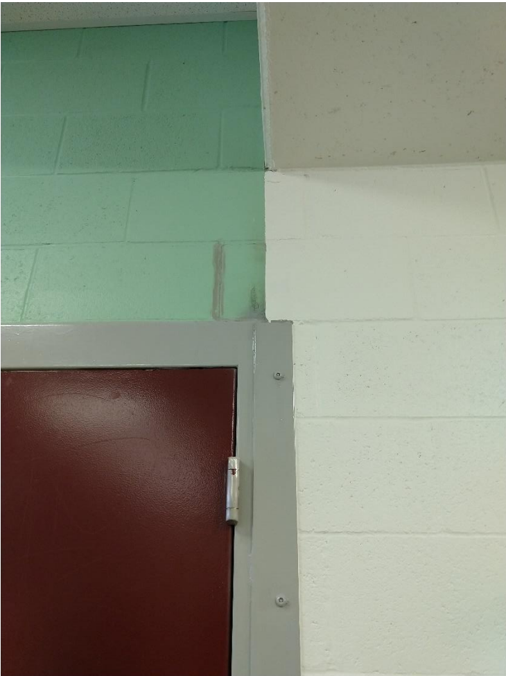
New Jail Addition - Unsettling
